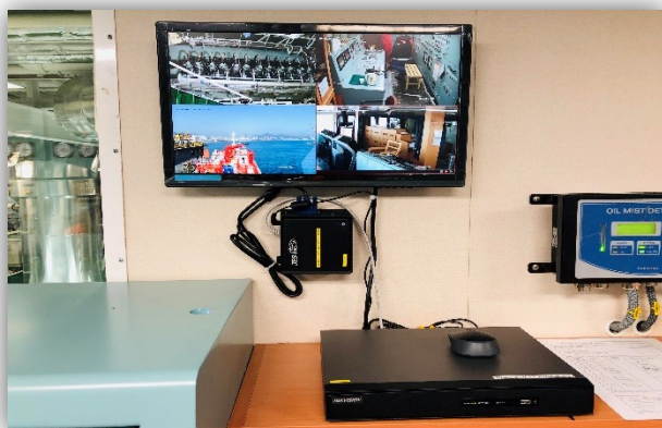
Engine Control Room
