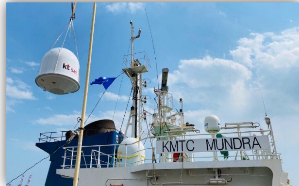
SATCOM System Buildup
