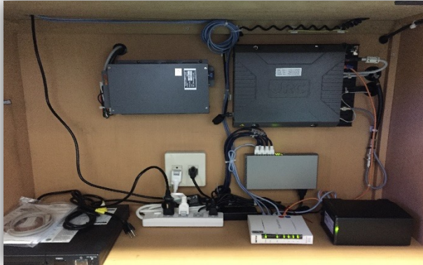
FBB/ NAS/ ROUTER/ FIRE WALL
